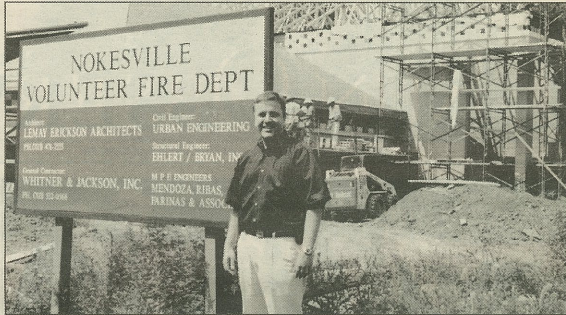
Construction is underway on a new station for the Nokesville Volunteer Fire Department and Rescue Squad station on Linton Hall Road, with a target completion date of Nov. 1. Jane Fullerton Lemons / the Bull Run Observer
